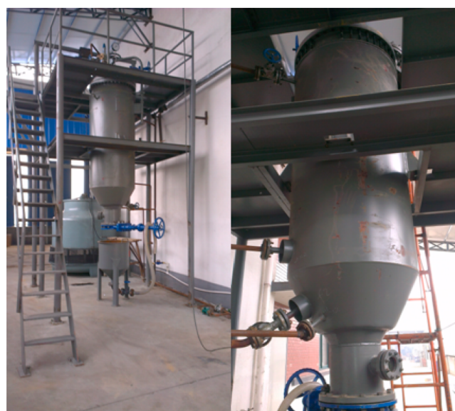
Figure 2. Image of the jacketed autoclave for disposal of pig carcasses.
